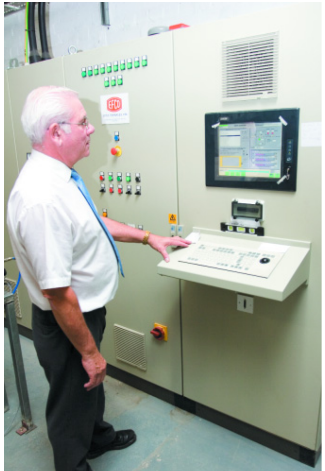
The upgraded graphical Windows based operator control station
